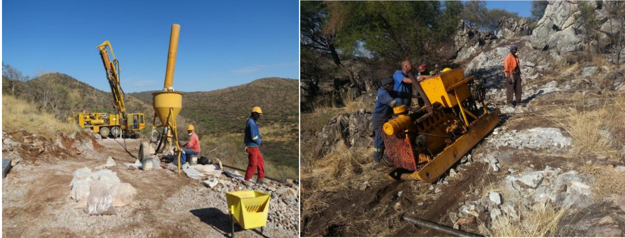
Figure 4. A truck mounted RC drill rig and a skid mounted drill rig (For illustration purposes)
