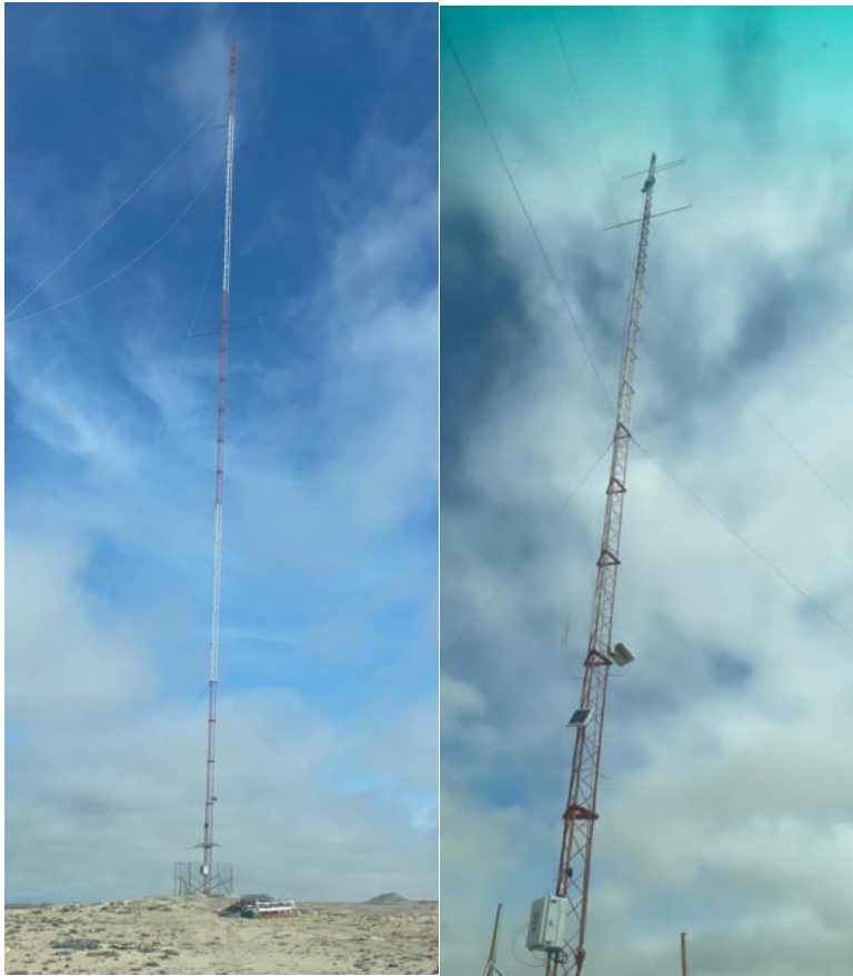
Figure 4 and 5 : Example of the NamPower Meteorological Wind Mast near Elizabeth Bay (67% complete at 67 m of 100 m).
