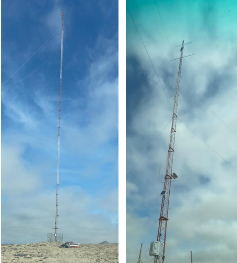
Figure 2 NamPower Meteorological Wind Mast near Elizabeth Bay (67% complete at 67 m of 100 m)
