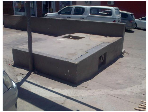
Photo 4. Existing oil-water separator
