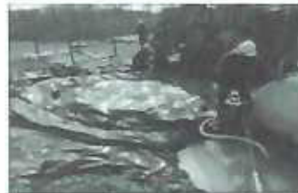
Sumps with plastic liner
