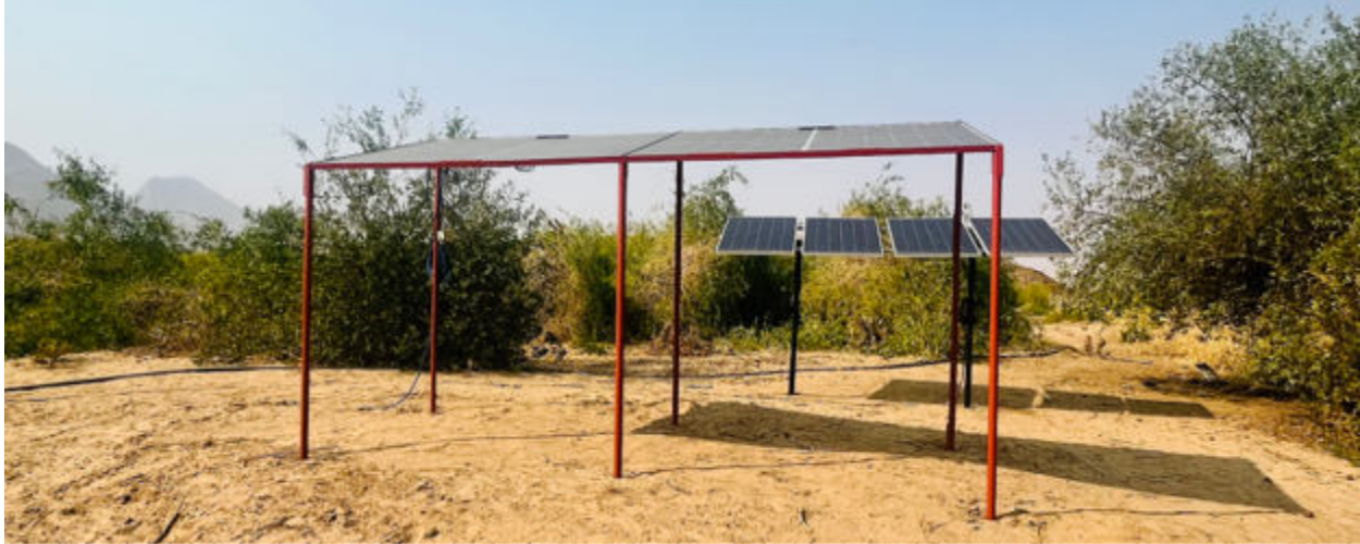
Figure 7. Existing Solar panel installations at project site
