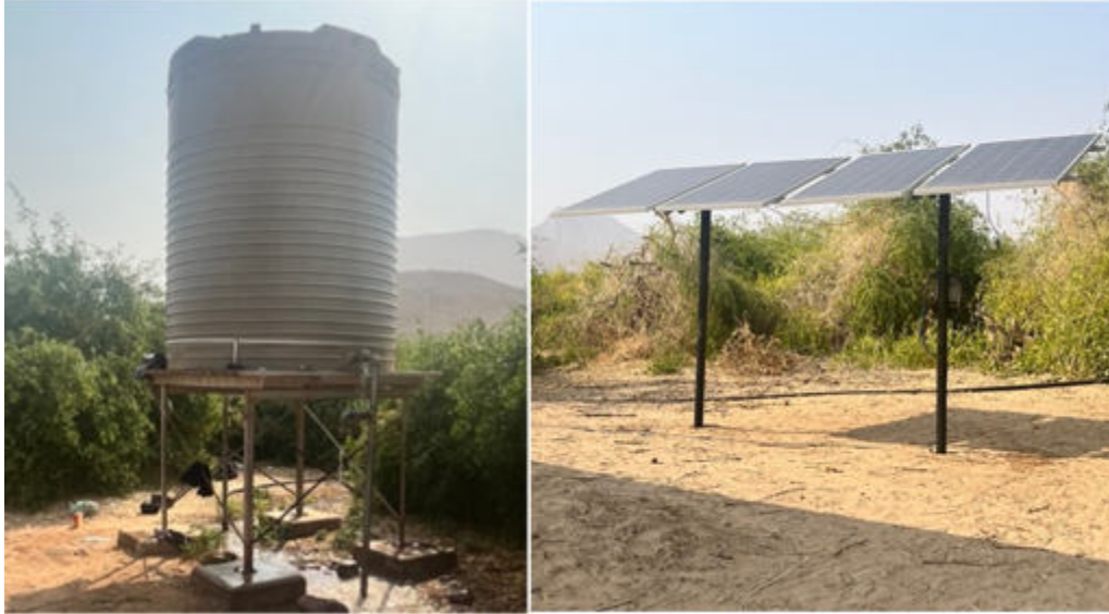
Figure 4. Water storage tank and solar panels for the conservancy office
