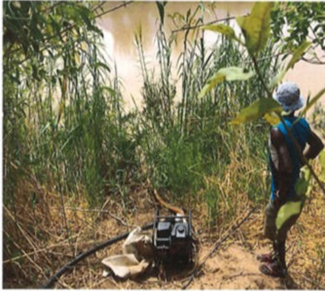
Figure 3. Generator used for water abstraction at Marienfluss Conservancy
