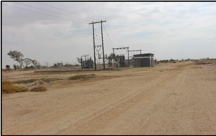
Figure 3: Arandis Sub Station and existing Servitude connecting to B2 Highway.
