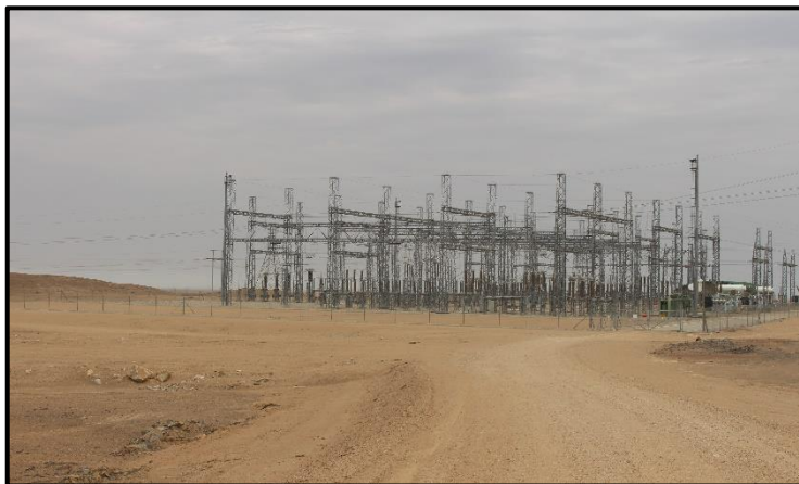
Figure 6: Existing Lithops Substation and access road to be used for OHL ROW
