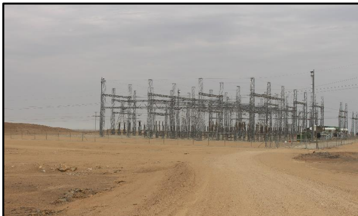
Figure 5: Existing Lithops Substation and access road to be used for OHL ROW
