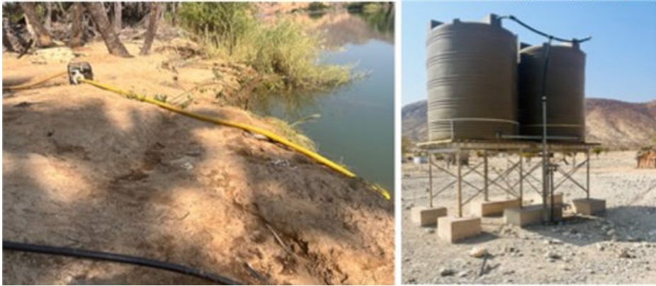
Figure 2. Diesel powered water pump and water storage tanks.
