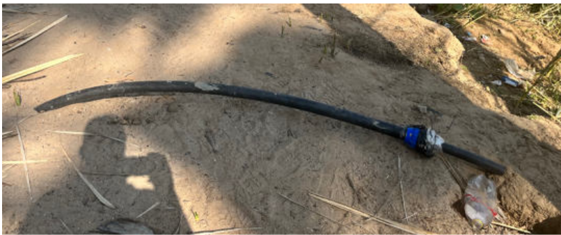
Figure 3. Broken water pipe aimed to supply water to the storage tanks.
