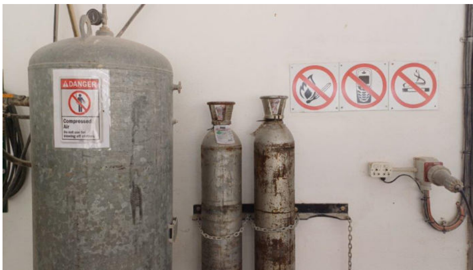
Photo 16 – View of warning signs at workshop.
