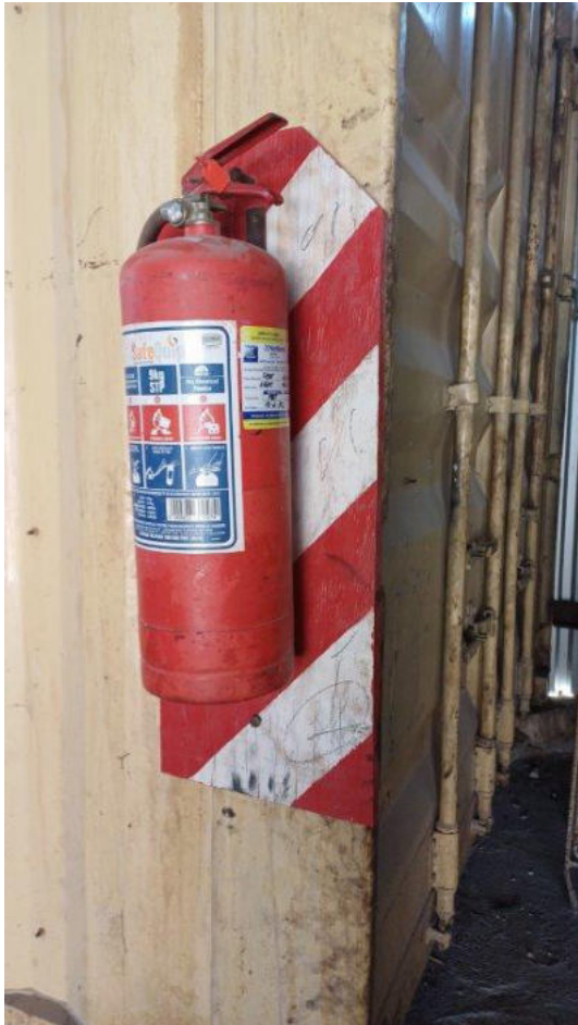
Photo 21 – View of fire extinguisher at personnel kitchen and eating area.
