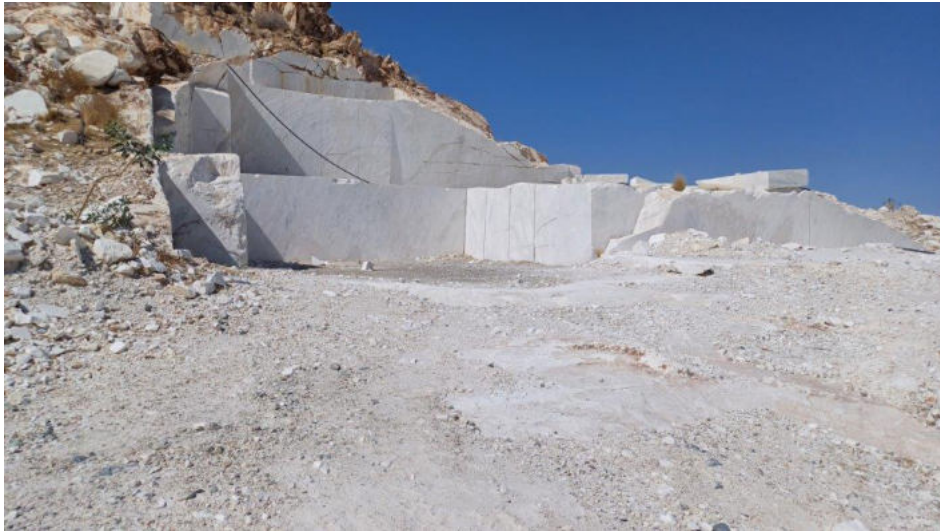
Photo 31 - View of one of the new test pits up the hill to the east of the main mining pit area.
