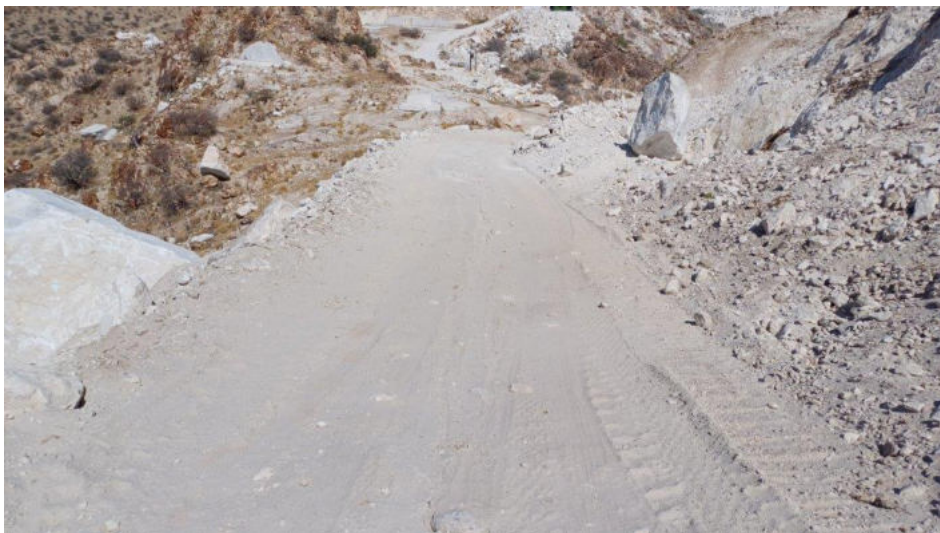
Photo 32 – View of the newly constructed road providing access to the newly opened test pits located to the east of the main mining pit area.
