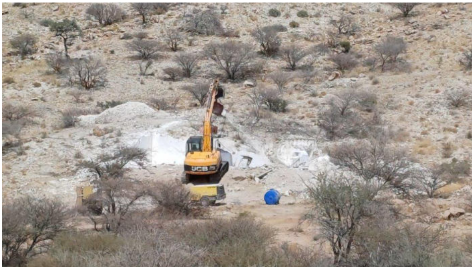
Photo 30 – View of new test pit located to the south-western edge of the larger mining area.
