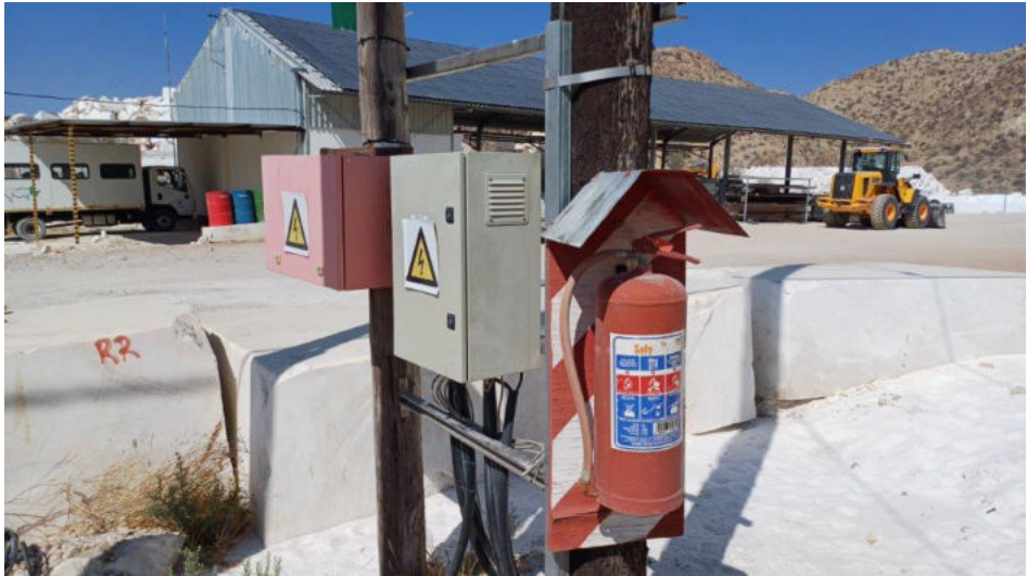
Photo 27 – View of fire extinguisher available on-site.
