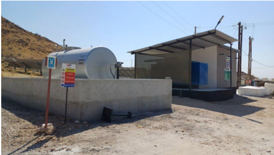
Photo 25 – View of newly constructed back-up generator and diesel storage area.
