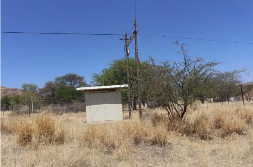
Figure 4: Power Box with electrical infrastructure
