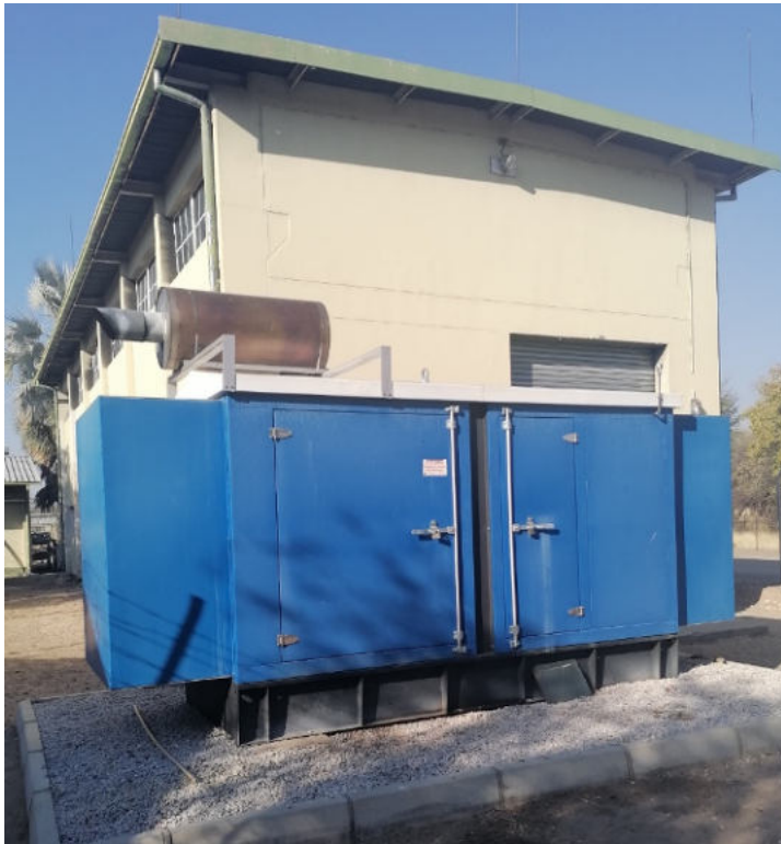
Figure 7: Back-Up Generator to the incinerator
