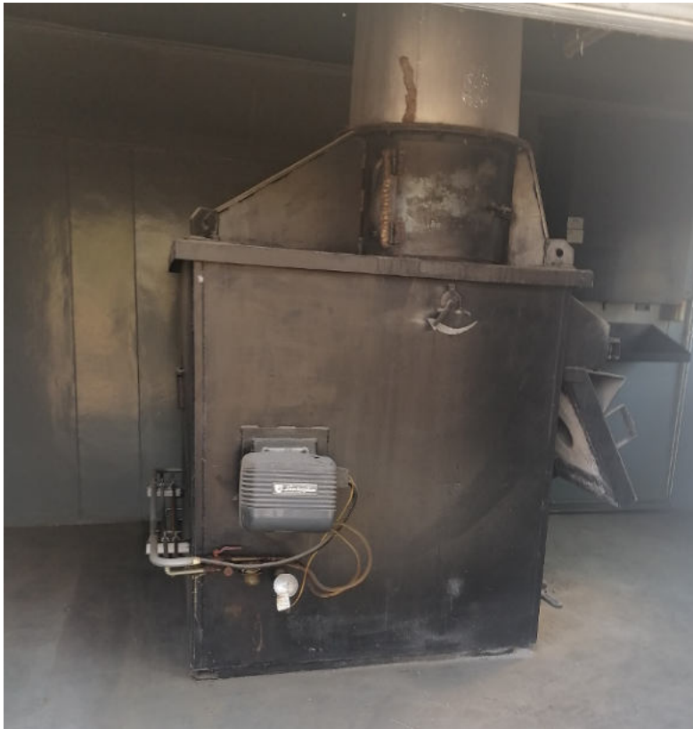
Figure 2. The Pathological incinerator at UNAM Ogongo Campus
