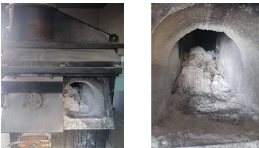
Figure 3. Burnt waste before disposal
