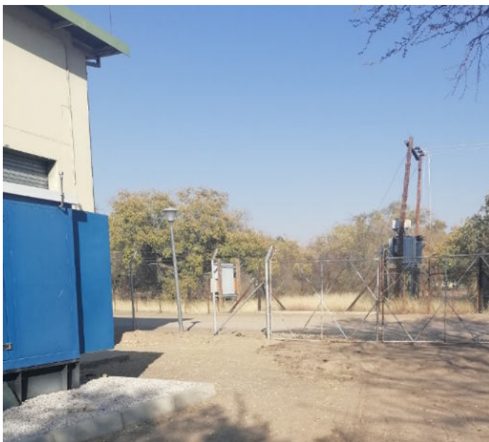
Figure 6: Grid Power Line for Ogongo Campus
