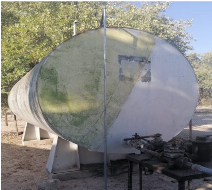
Figure 4: Shows a 1000L capacity diesel tank that feeds the incinerator
