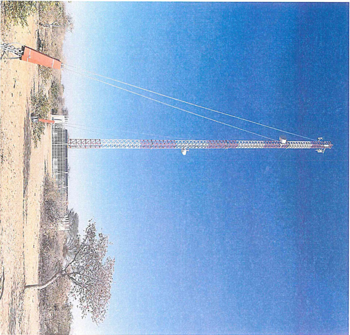
Full tower with 3x Panels antennas and two MW dishes
