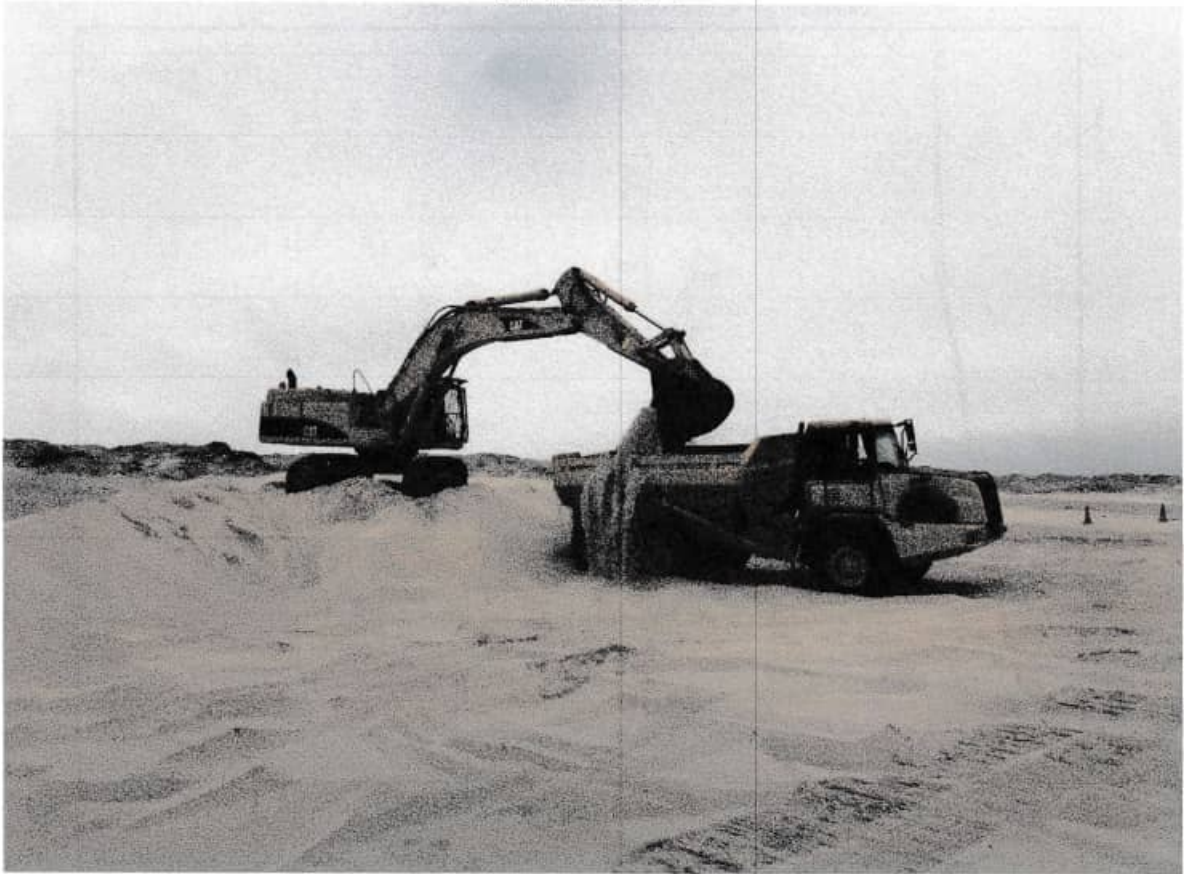
Earthmoving equipment on site and in operation at NNDC. (Source: Johan van Rooyen – NNDC Manager)
