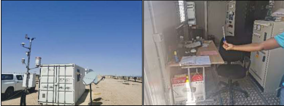
Figure 2-2: Fully equipped control rooms (offices) for the Solar Park Site
