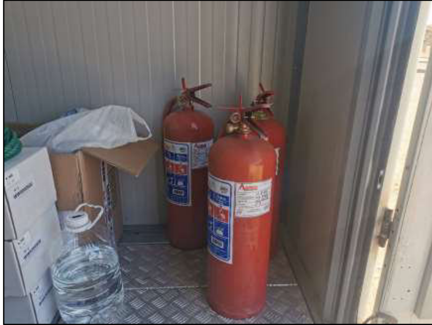
Figure 2-8: The three site fire extinguishers inside the control room (office) onsite
