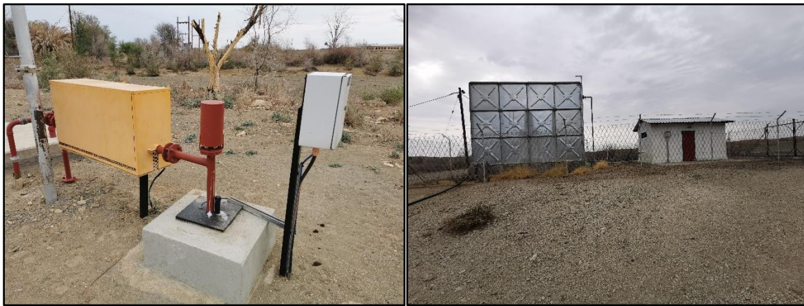
Figure 24: One of the NamWater boreholes (left) and Tses Village Council borehole observed to the east of the existing sewer ponds
