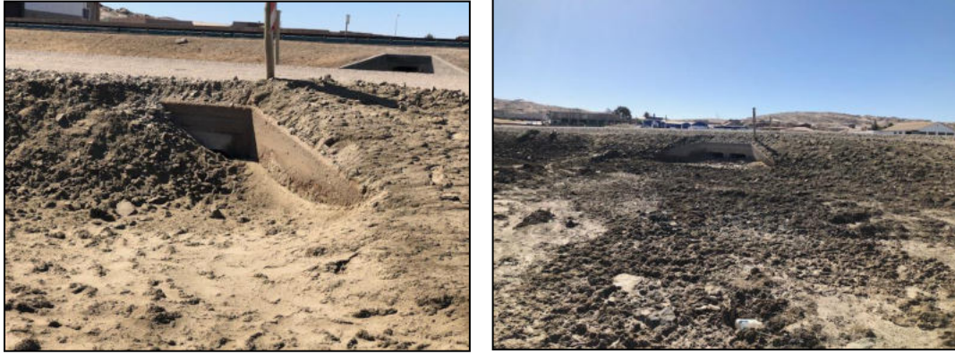
Figure 10: Culverts dumping surface water from surrounding areas onto the site
