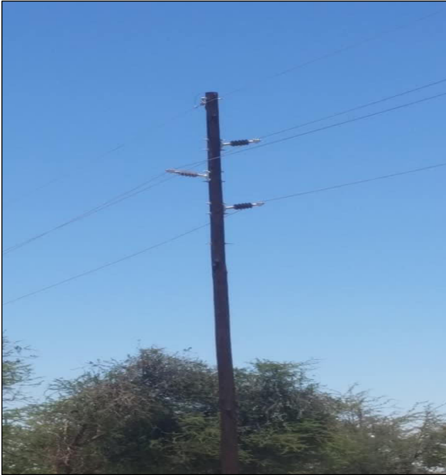
Figure 4: Typical 11kV power line structure
