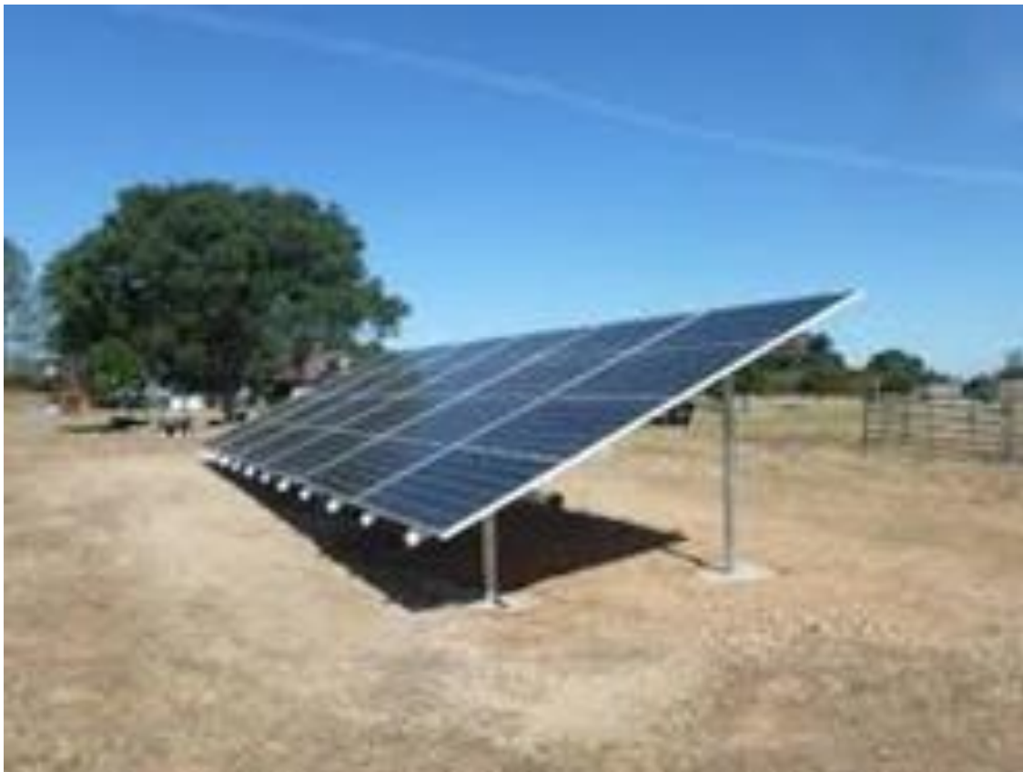
Figure 3: Typical mini-solar plant (photo for illustrative purposes only).
