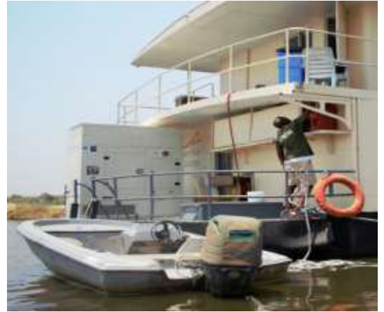
Figure 3 Location of generator at back of the houseboat
