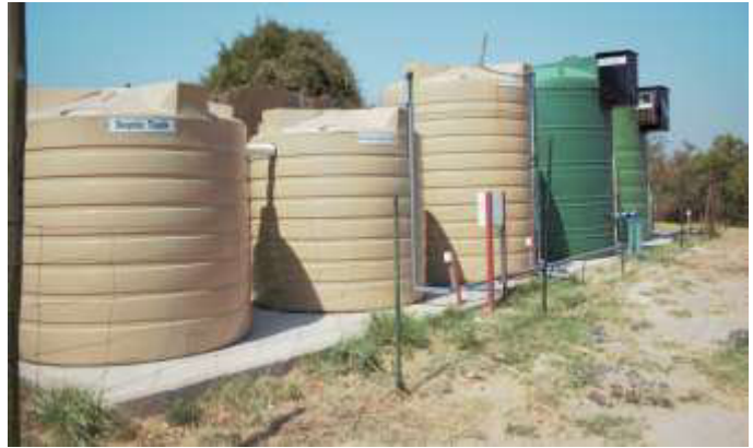
Figure 8 Effluent treatment system at Ncheku-Kasika
