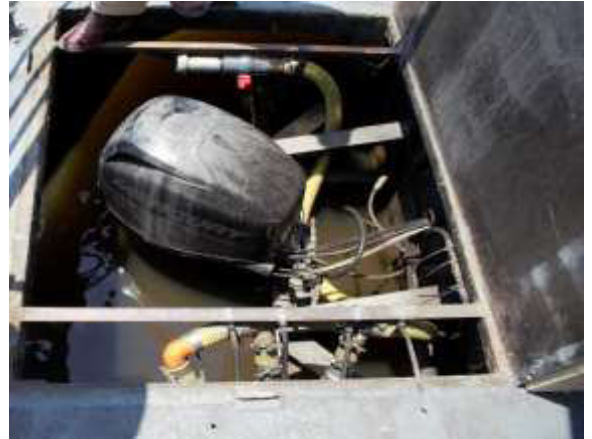
Figure 5 Piping for pumping effluent off the houseboat's tanks
