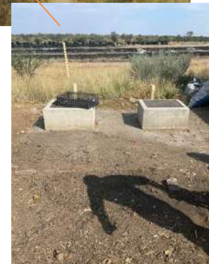
Soak away sewer reticulation system, serving plant and residence.
