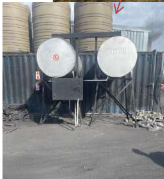
fuel storage facility, bunding needed ASAP!
