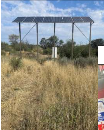
Borehole site and Solar panels for water supply to plant and ablutions.
