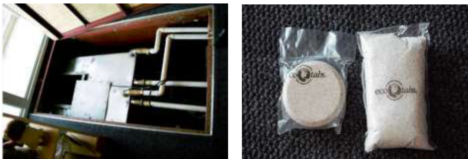
Figure 5 First sewer tank onboard the houseboat where eco-tabs are applied
