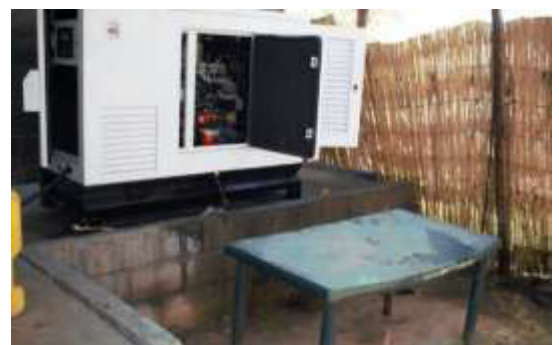
Figure 14 Diesel generators for power supply for onshore operations and overnight to Zambezi Queen houseboat
