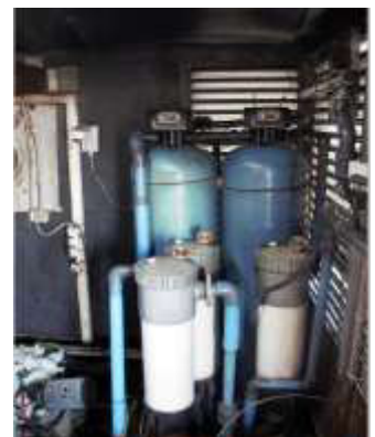
Figure 3 Treatment of water for facilities and ice making machine
