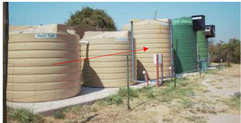
Figure 9 Effluent treatment system at Ncheku-Kasika
