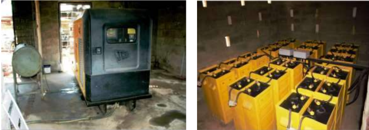
Figure 2 Outlook of the generator room with rechargeable batteries for the solar power system
