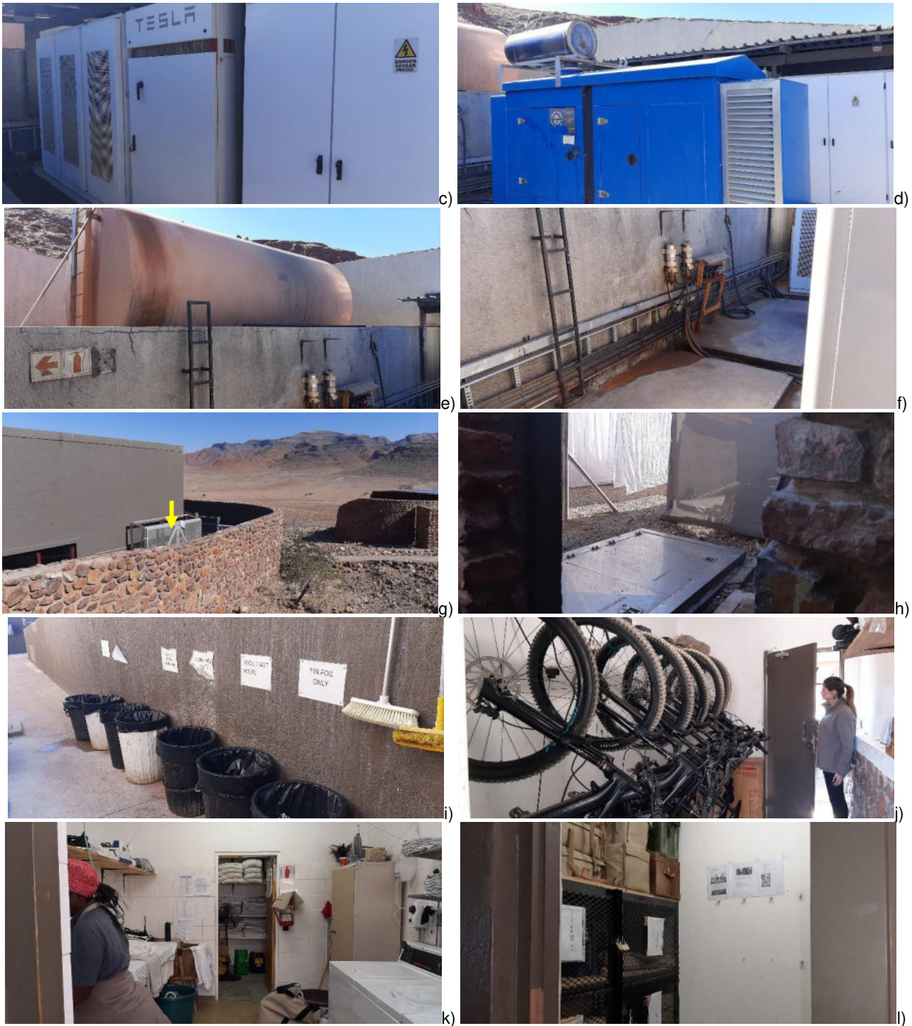
Figure 7: Pictures showing: a) solar panels on the back-of-house area; b) back-of-house; see the cage with gas bottles (yellow arrow); c) the batteries, inverter, and distribution board; d) 250 kilo Volt-Ampere (kVA) generator; e) and f) consumer fuel installation; g) and h) area with cage with gas bottles, laundry lines, and the fat trap; i) an area for waste segregation; j) e-bikes; k) the laundry; and l) store room for the guides (Source: L Maartens, July 2023).
