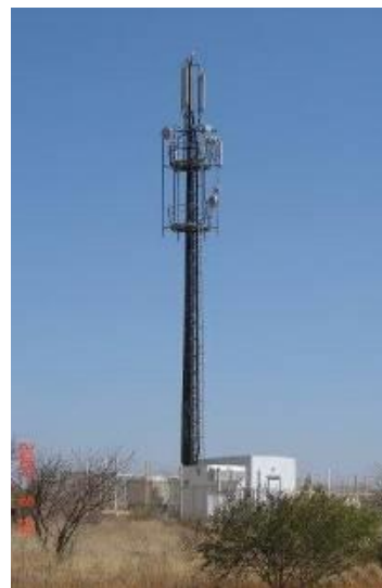
Figure 5-4: Example of BTS (Monopole)
