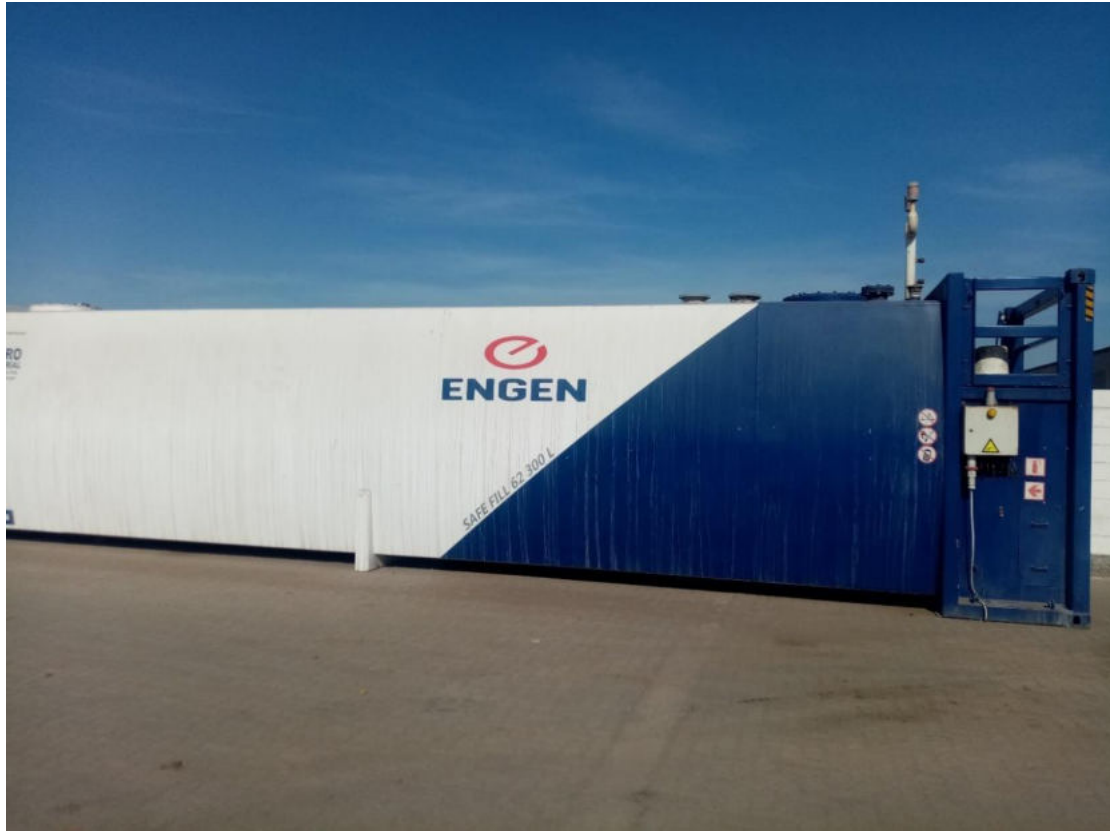
Figure 1: Self Bunded Engen 62 300 L tank
