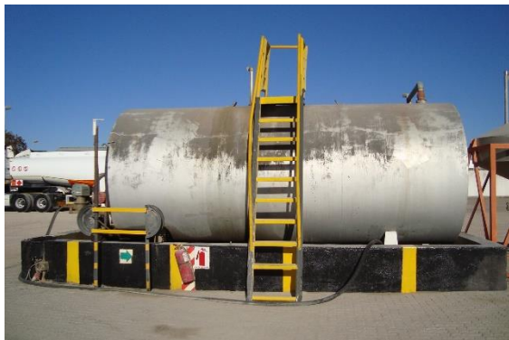
Photo 4-1. Diesel storage tank in bund area
