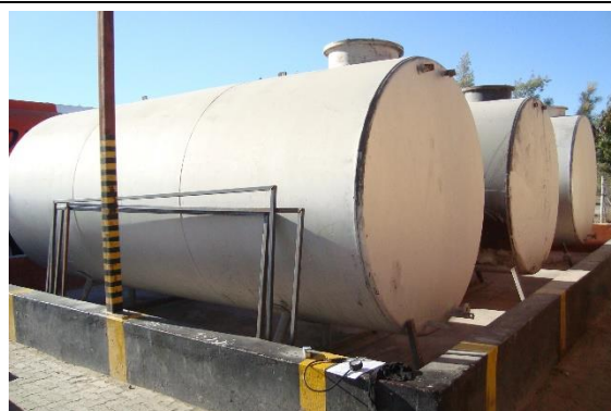
Photo 4-6. Contaminated fuel tanks (not used)
