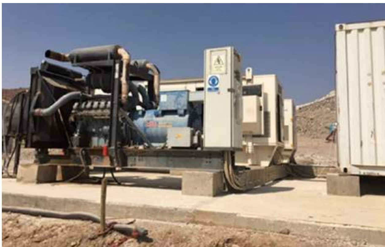
Figure 22 - Genset stand-by power source (Source: Minxcon, 2021)
