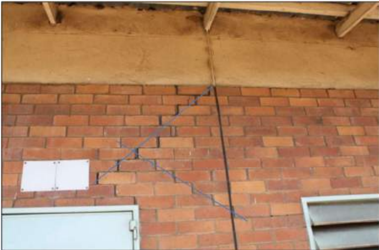
Figure 8: Example of blast induced damage.
