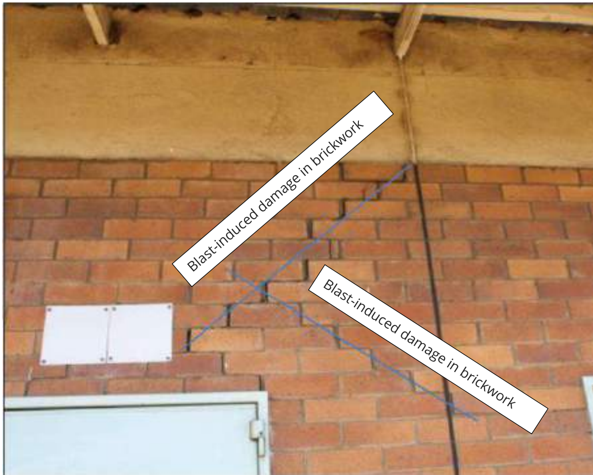
Figure 15 – Example of blast-induced damage
