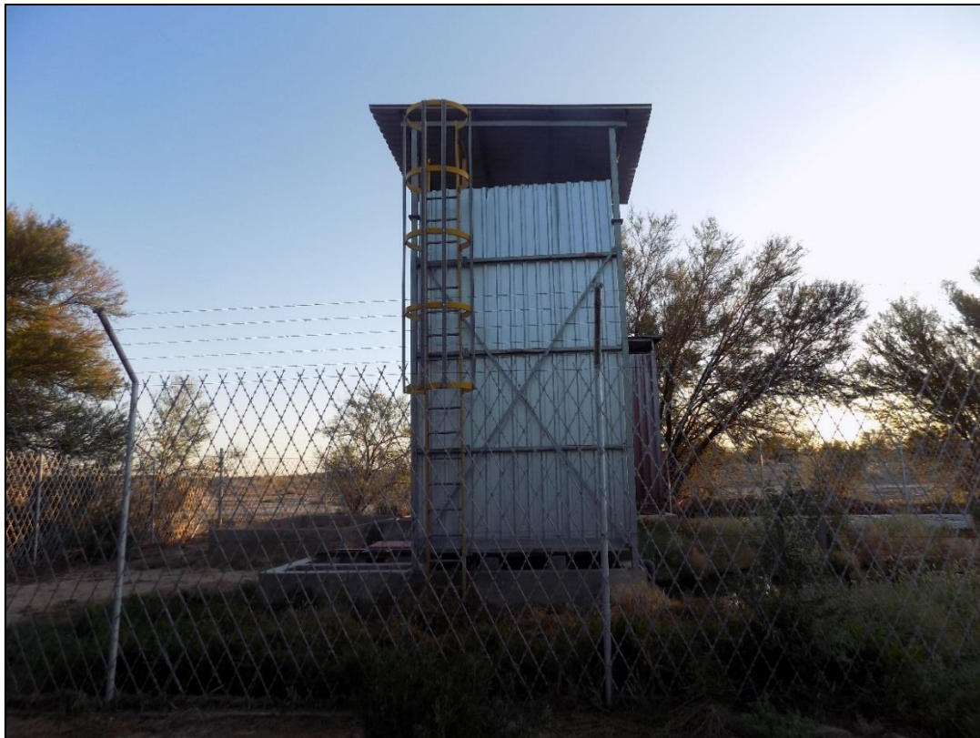
Figure 1-3: Wastewater Treatment Plant
