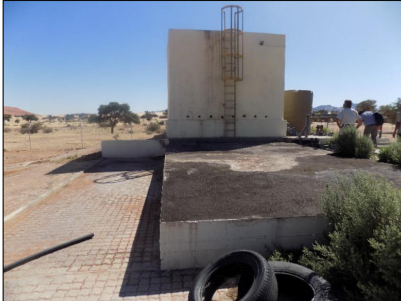
Figure 1-4: Waste water Treatment Plant
