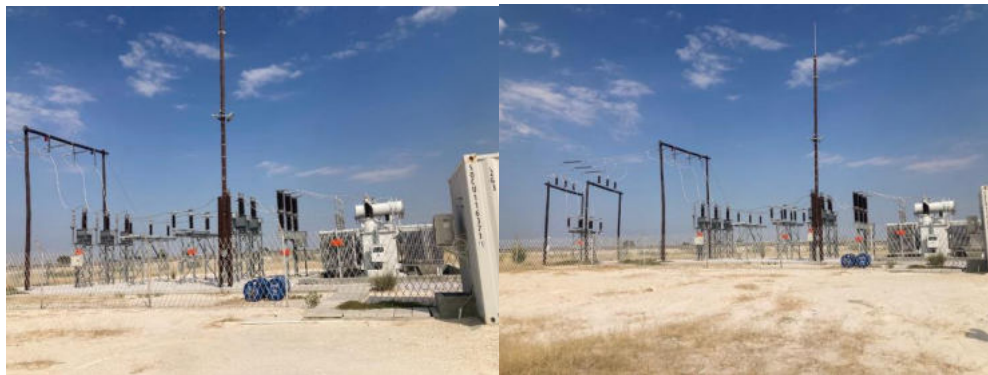
Figure 2-2: The site substation (associated infrastructure) connecting the Site to the NamPower Substation
