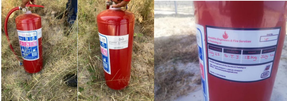
Figure 2-7: One of the five site fire extinguishers onsite
