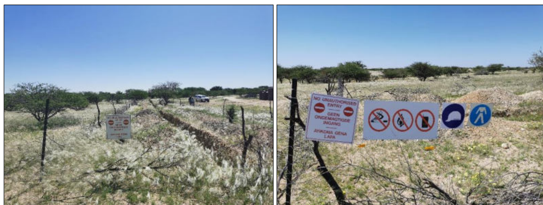
Figure 2-4: Fenced off exploration trenches awaiting backfilling upon completion of sampling (photos taken at a precious metals exploration site visited by the Author in Erongo Region)
