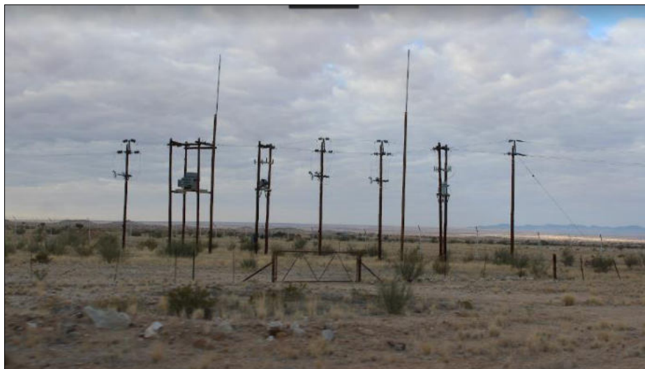
Figure 5-16: One of the power grid powerlines in the area
