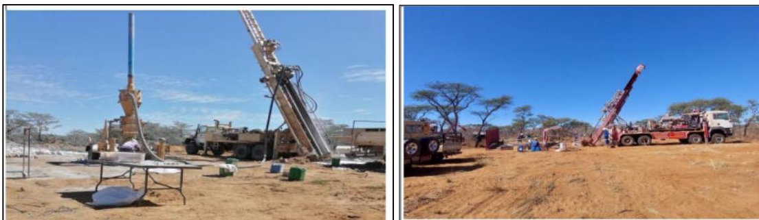
Figure 2-3: A drill rig at an active EPL in the Omaheke Region (Resilient Environmental Solutions, 2022)
