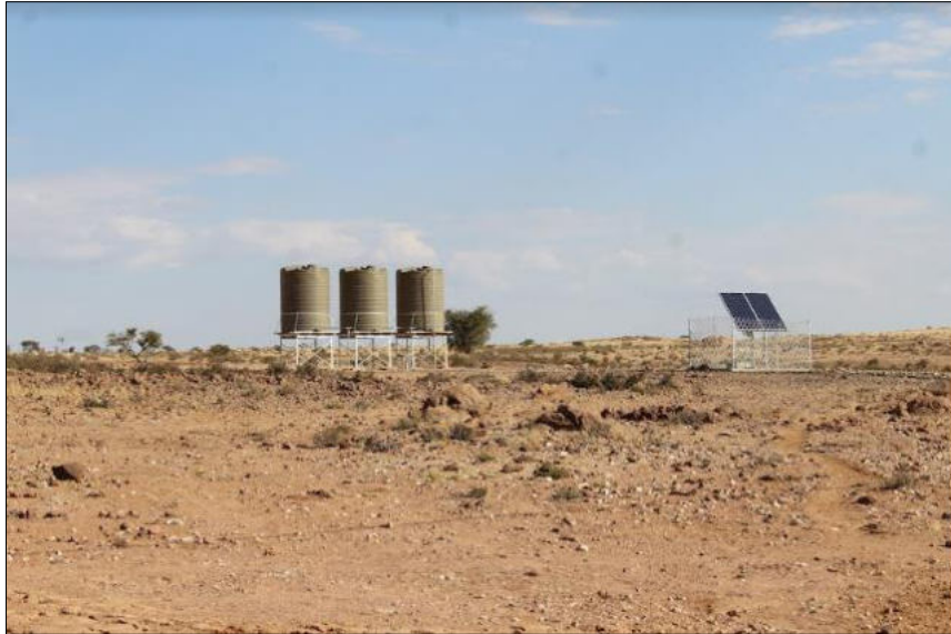
Figure 5-15: Some of the water storage tanks supplied by a solar powered boreholes at Warmbad
