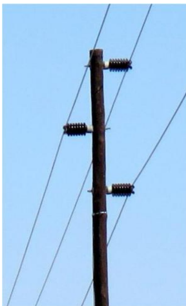
Figure ii Example of "gapping" of vertical earth wire on 11 horizontal line post compact delta (HLPCD) pole (arrow shows upper limit of the earth wire).
