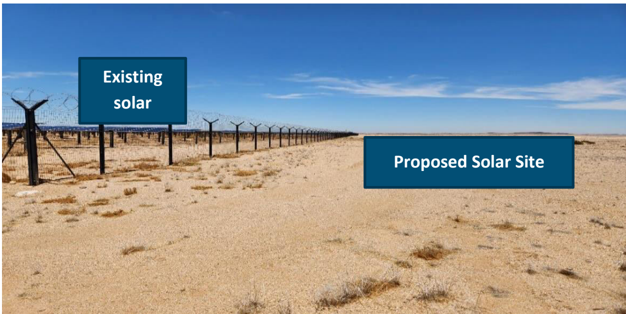
Figure 4: Laying foundation: The structures will be connected to the ground through metal screws. The exact method will depend on the detailed geotechnical analysis
