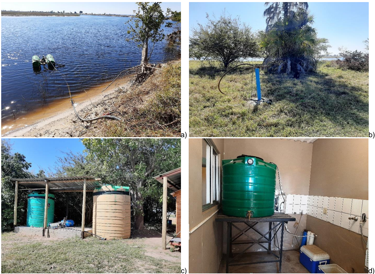
Figure 9: Pictures showing: a) water abstraction from the Chobe River; b) water supply borehole; c) two water storage tanks; and d) the potable water filtration system (Source: L. Maartens, 02 July 2020).
