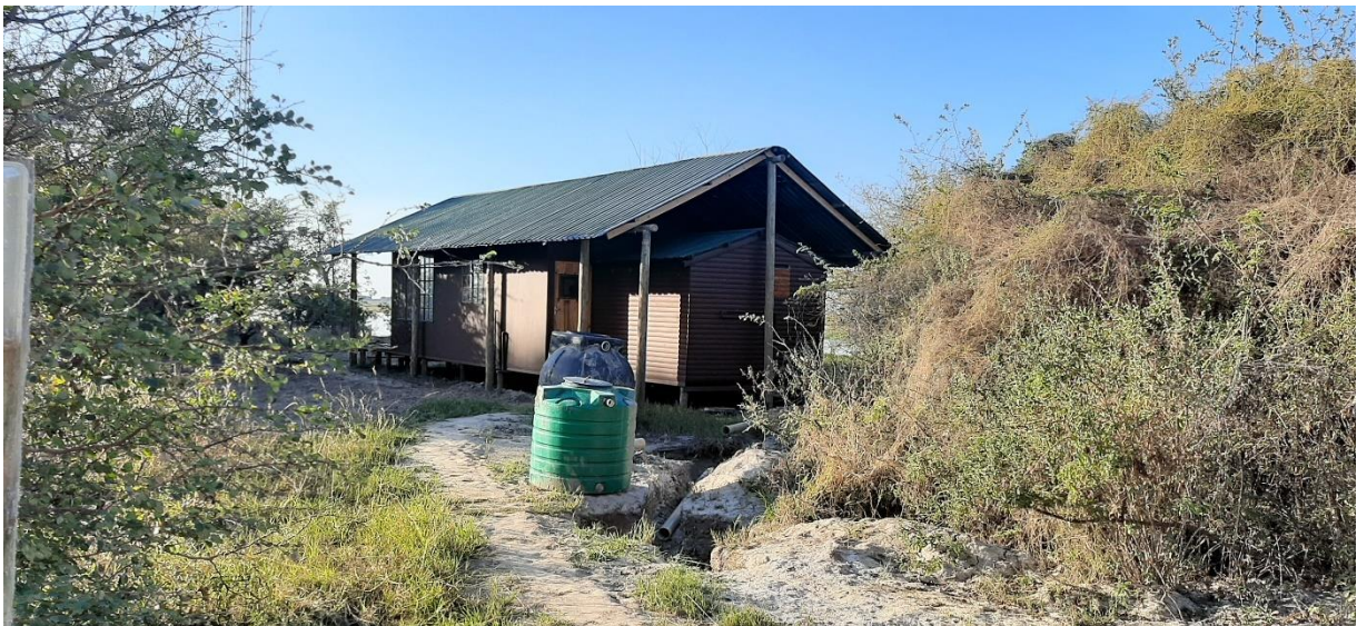
Figure 6: Picture showing the Assistant Manager's house (currently under construction) (Source: L. Maartens, 03 July 2020).
