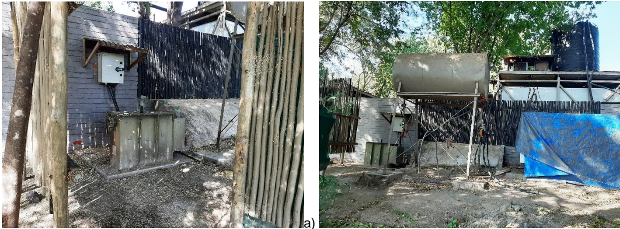
Figure 10: Pictures showing: a) transformer; b) fuel tank and diesel generator (Source: L. Maartens, 02 July 2020).
