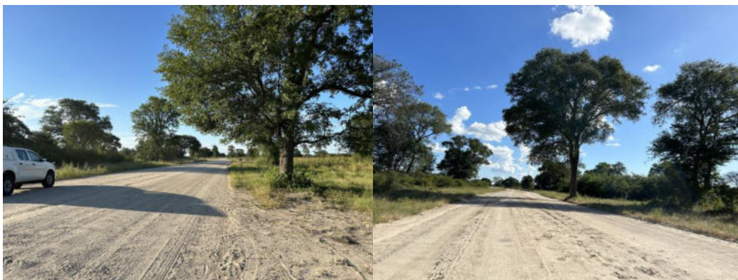
Figure 1: The current condition of the gravel roads with some sections being too flat and susceptible to flooding when it rains.
