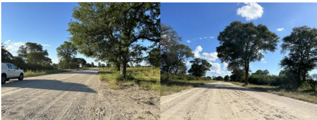
Figure 1: The current condition of the gravel roads DR3507 & DR3559 with some sections being too flat and susceptible to flooding during rainy season.
