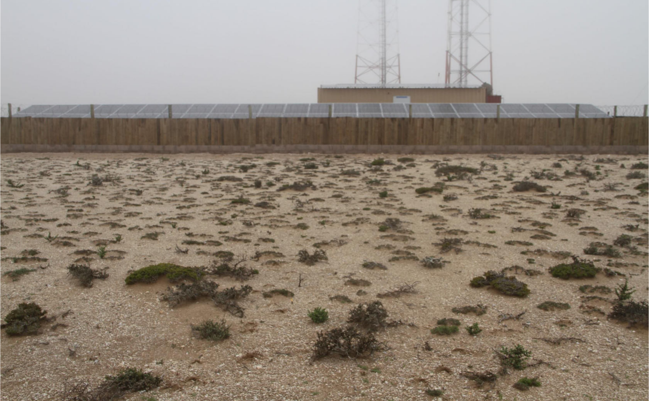
Plate 1.4: Existing infrastructure, solar PV Park that supplies power to the Kerbehuk line of sight communication station.
