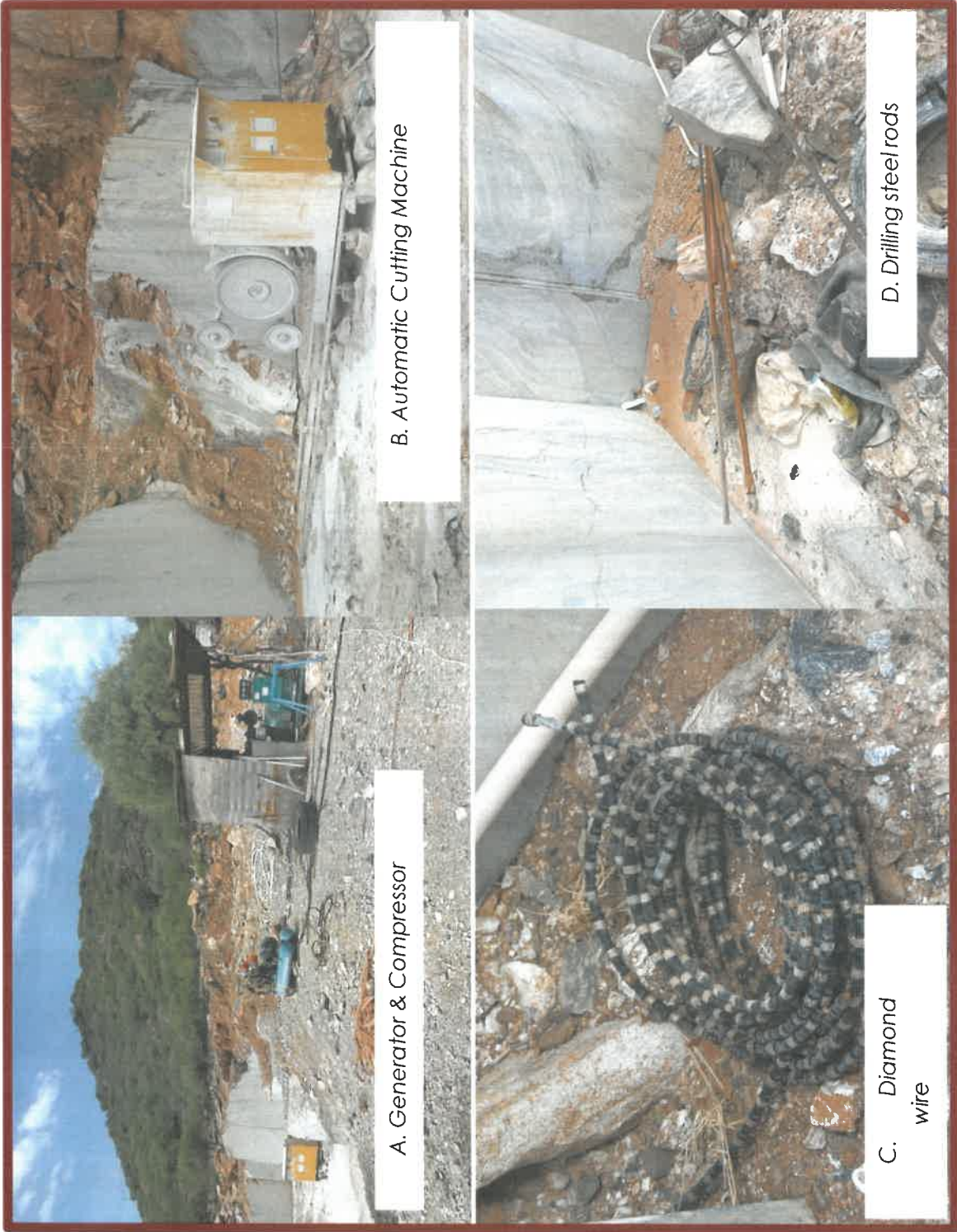
Figure 9: Minerals will be extracted using an automated diamond wire machine to produce the commercial grade cubes (HEEC, 2023- Illustrative pics)
