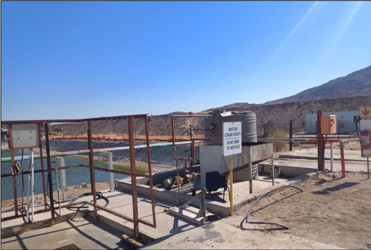
Photo 1: Process pond to be repaired
