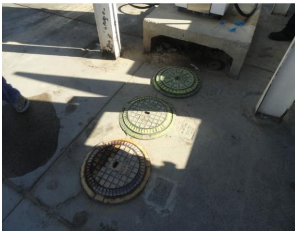
Photo 3. Filler point containment
