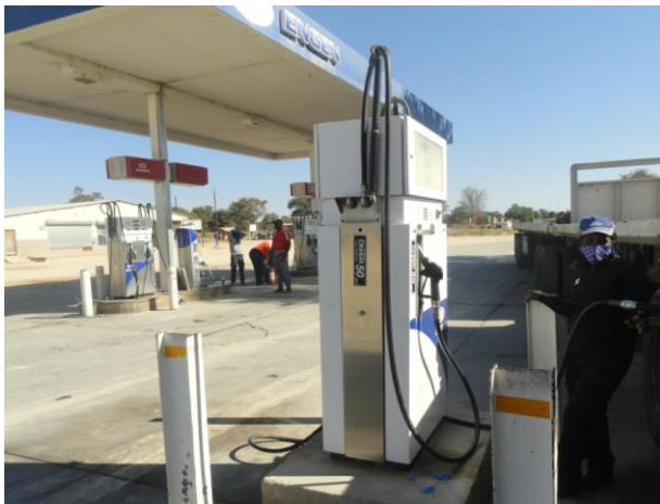
Photo 2. Existing dispensing points on site
