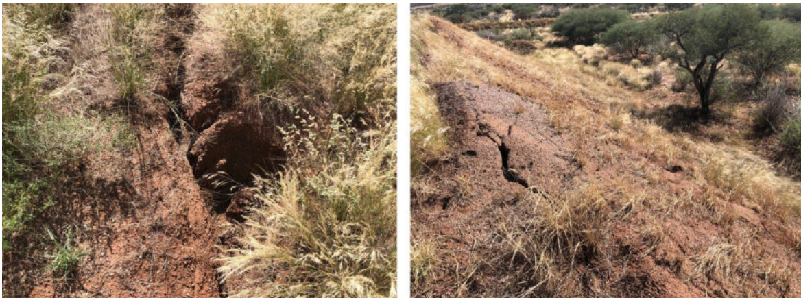
FIGURE 13: GULLY EROSION ON THE REJECT DEPOSITORY
