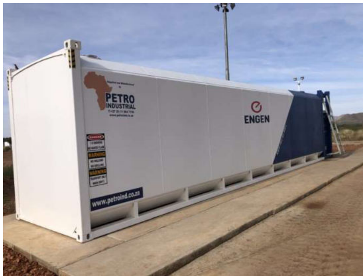
FIGURE 9: THE DOUBLE-CONTAINERIZED FUEL TANK FACILITY OF ENGEN ONSITE
