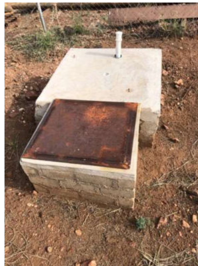
FIGURE 5: FACILITY FOR THE CONTAINMENT OF SEWAGE
