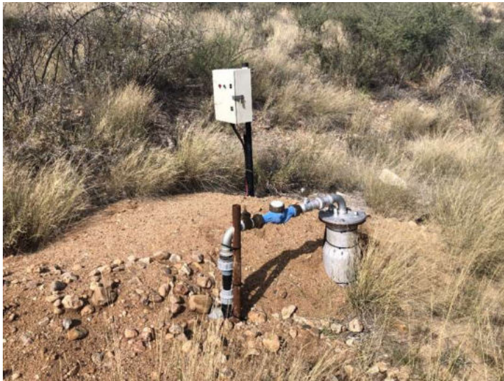
FIGURE 6: ONE OF THE ABSTRACTION BOREHOLES
