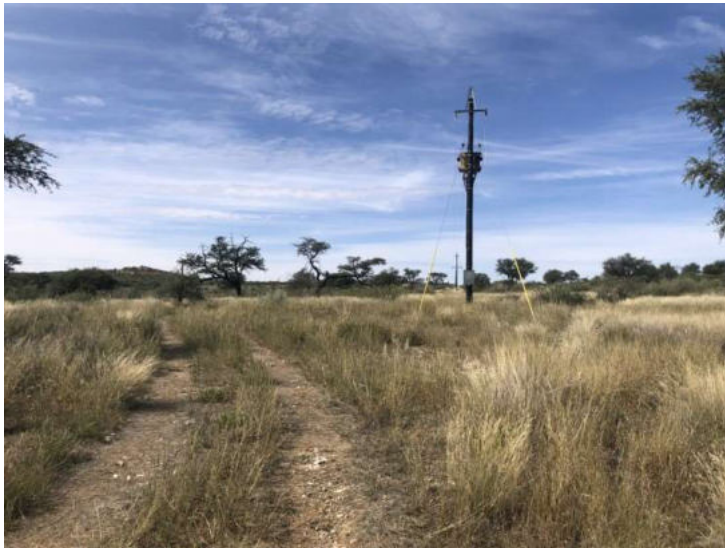
FIGURE 8: THE POWERLINE THAT PROVIDES ELECTRICITY TO THE ABSTRACTION BOREHOLES
