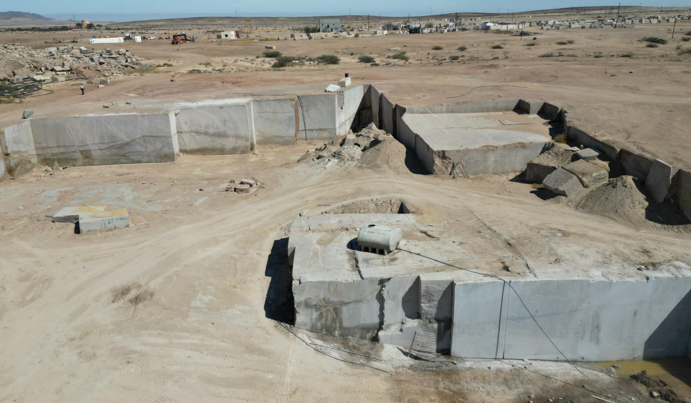
Plate 1.2: Detailed overview a granite quarry operational area, stockpile, sorted waste blocks for reuse and workshop and processing operations.
