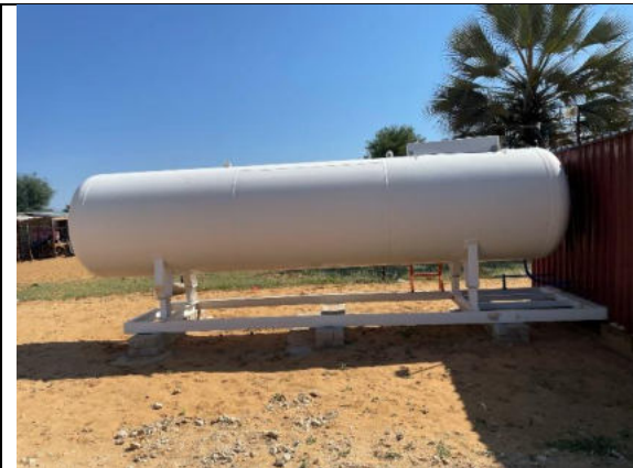
Photo 4-1 LPG storage tank
