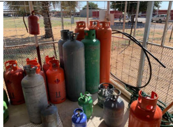
Photo 4-2 LPG cylinder storage area
