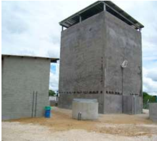
Figure C4a): Trickling filter tower
