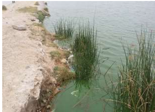
b) Damaged embankment and growth
