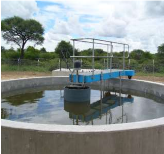
Figure C5: Clarifier with Rotating Bridge
