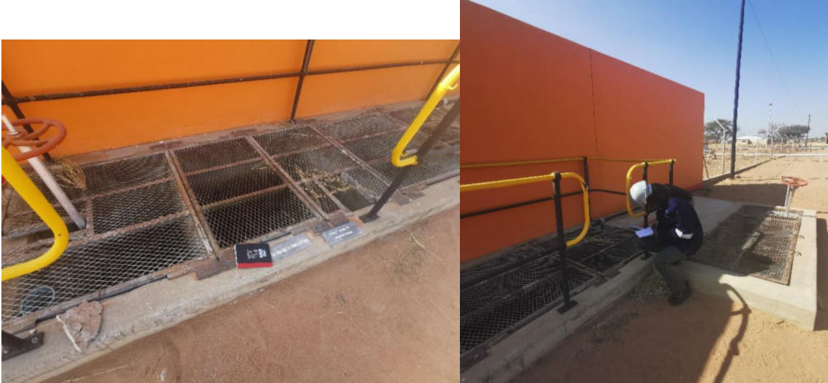
Figure 2-9: The oil-water separator onsite
