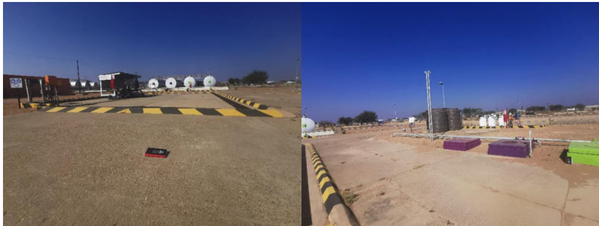
Figure 2-8: The concrete lined gantry at the aboveground and underground fuel tanks areas
