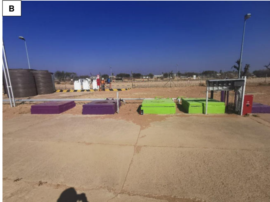
Figure 2-1: A - The above ground tanks and B-marked covers of the underground tanks onsite
