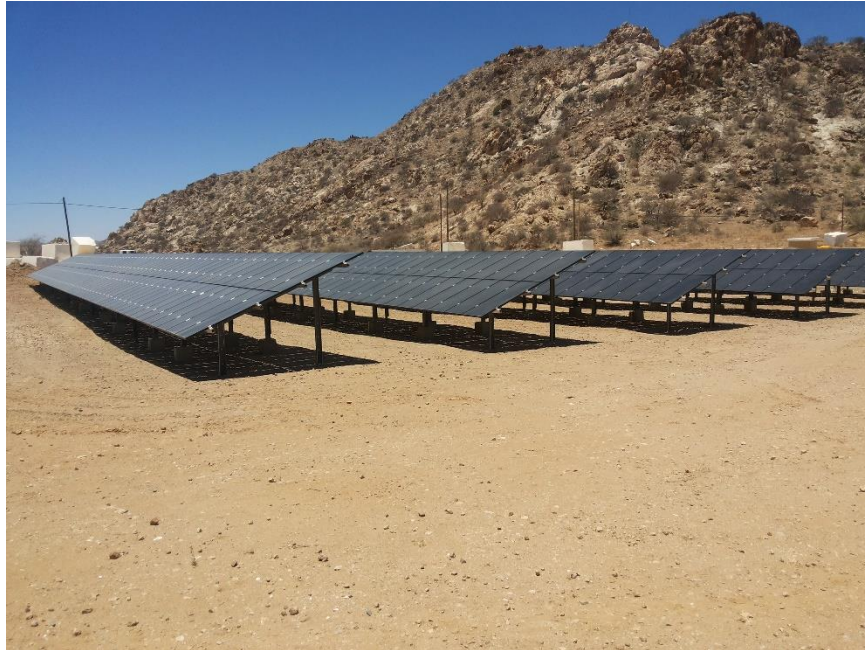
Figure 9: View of a section of the Solar Plant
