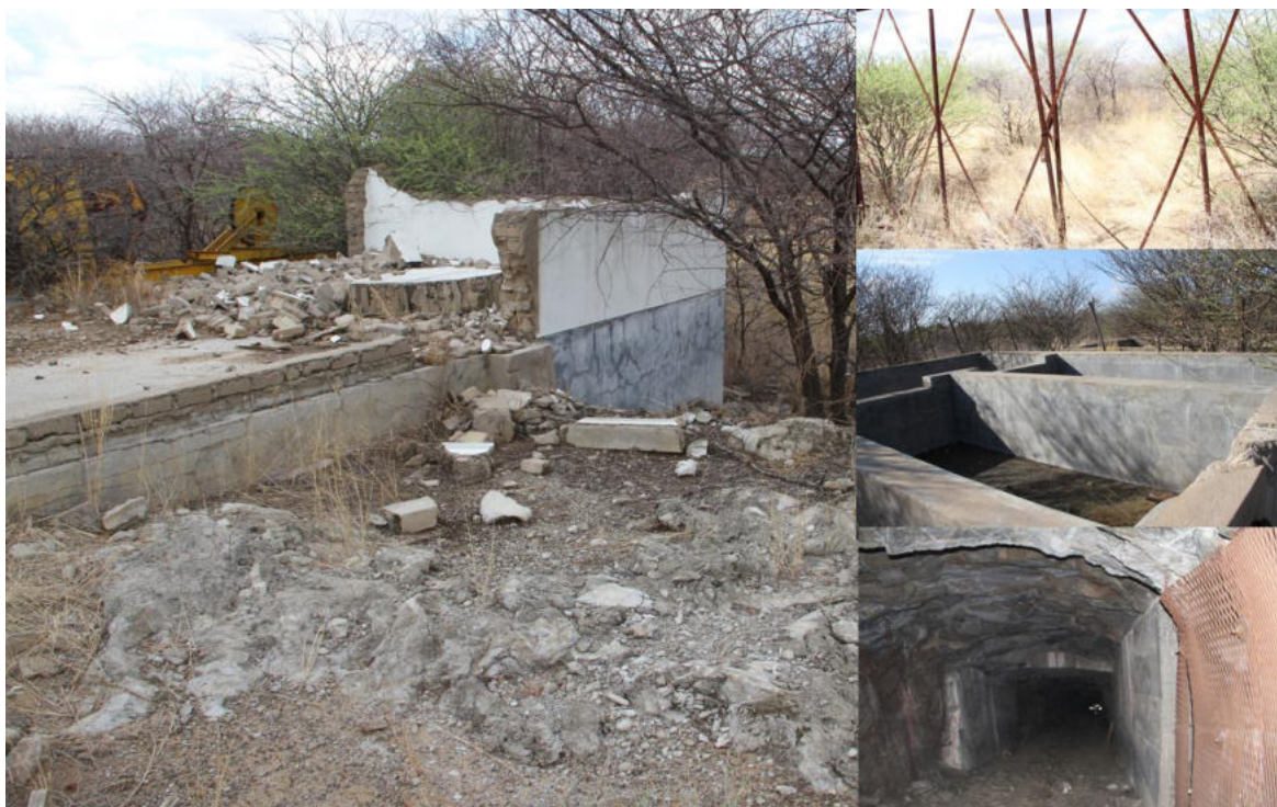
Plate 4.5: Old unstable structures, old fences / gates, mineral processing and services all found around Farm Elbe No. 10.
