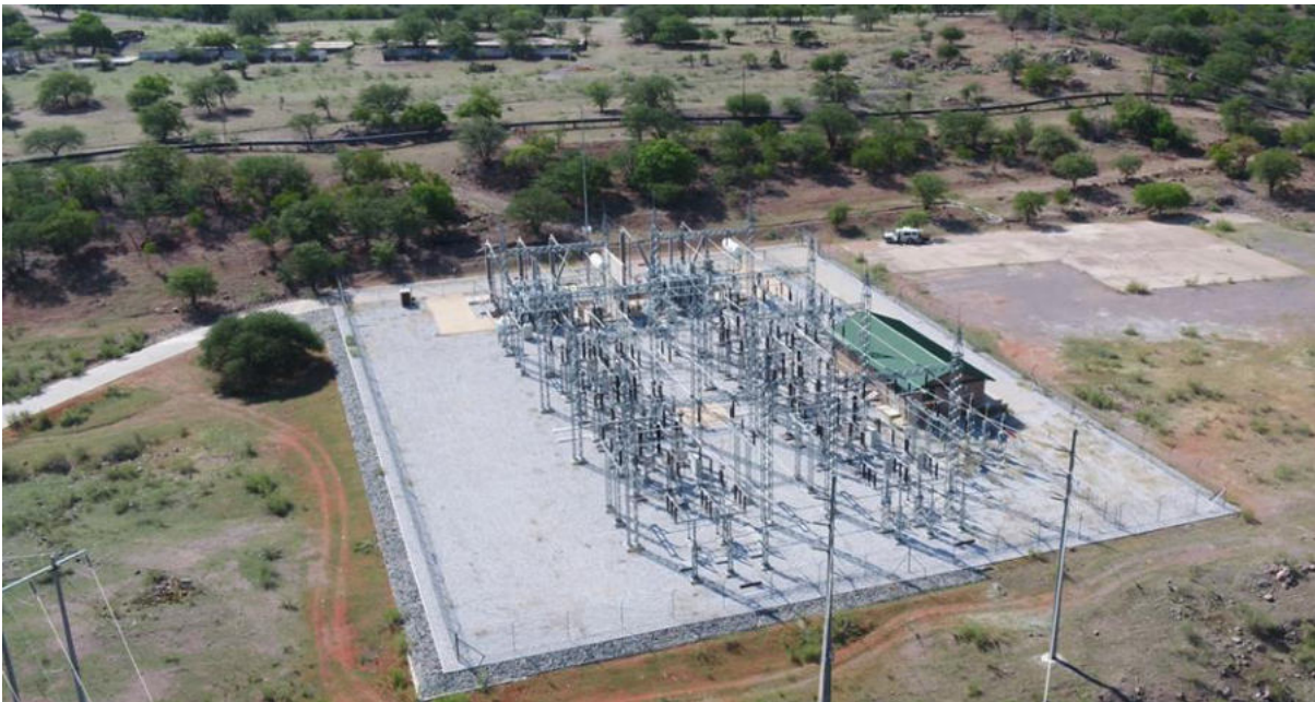
Figure 3: Hippo station also clear of litter (picture taken during drone inspection and surveys)
