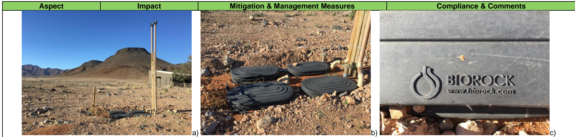
Figure 11: Pictures showing: a), b) and c) staff village Biobox sewage plant system; and d) (Source: Mr Andrew Schoeman, Back of House Manager & BEYOND).
