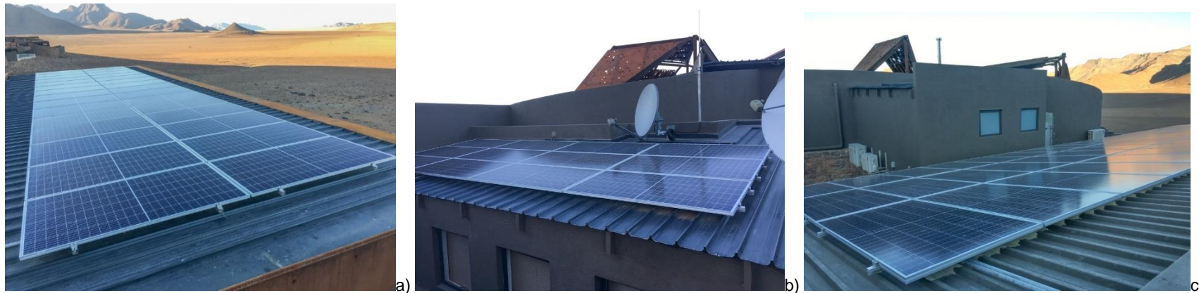
Figure 8: Pictures showing: a) guest suite solar panels; b) solar panels above the office; and c) solar panels above the kitchen (Source: Mr Andrew Schoeman, Back of House Manager &BEYOND).
